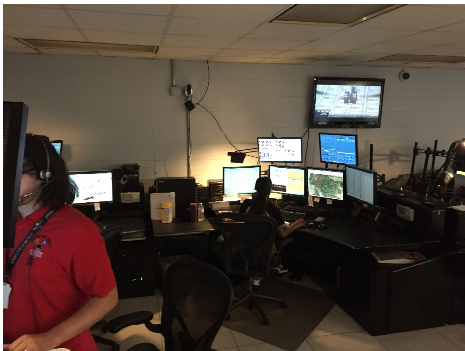
Figure 8: View of Console Workstation (2)
